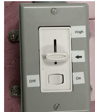
Figure 2 Heater control switch
